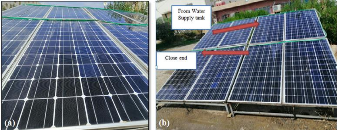
Figure 2: a- Cooling pipe installation, b- Cooling pipe installation on the PV array
