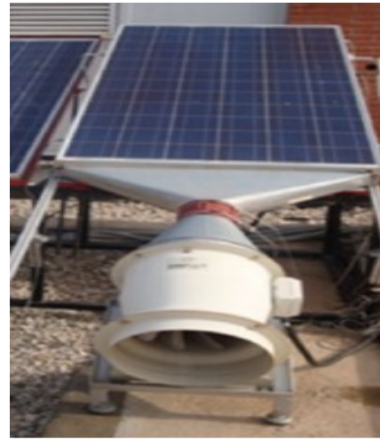
Figure 3. Shows the forced convection air cooling [19].
