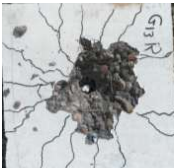
Fig. 11. Crack Patterns ( reference mix )
