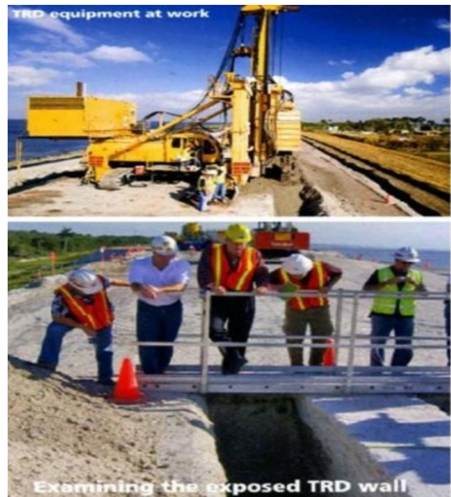
Figure 9. Top: TRD machinery in operation; Bottom: TRD wall inspection at Herbert Hoover Dike, which encircles Lake Okeechobee in southeast Florida[18]
