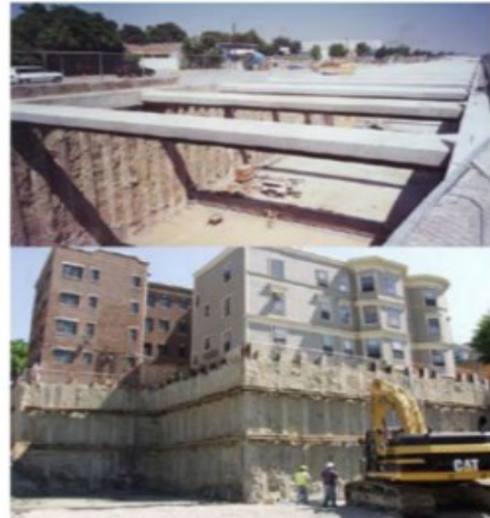
Figure 11. Above A railroad trench excavating job for the Alameda corridor. Bottom: A structural cutoff wall built during the building of a new Harvard University building in Cambridge[18]
