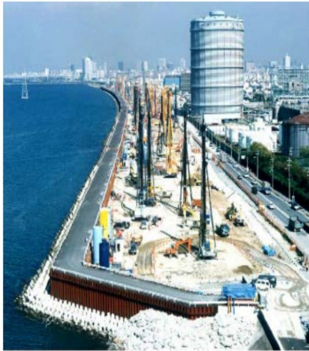
Figure 13. Application of DJM and resulting columns at Yodogawa River embankment in Japan(18)
